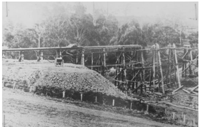
Building the big trestle bridge near Strzelecki Image; On display at the Back-to Bayles celebration in June 2022
